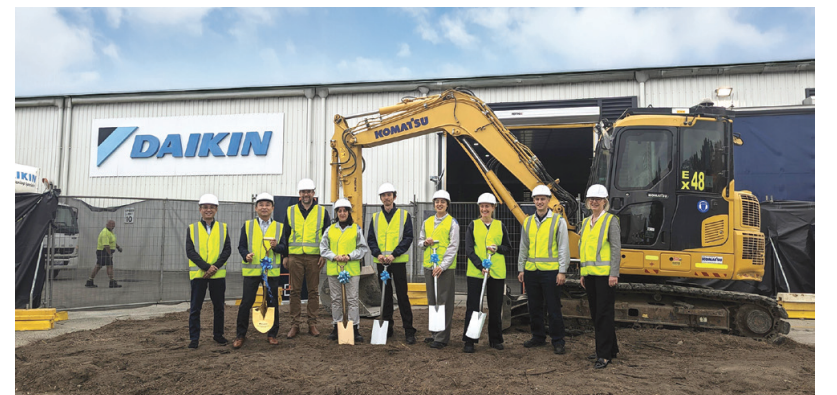
Daikin Australia's state-of-the-art manufacturing facility in Sydney continues to expand to drive advances in energy efficiency and in-home comfort.
