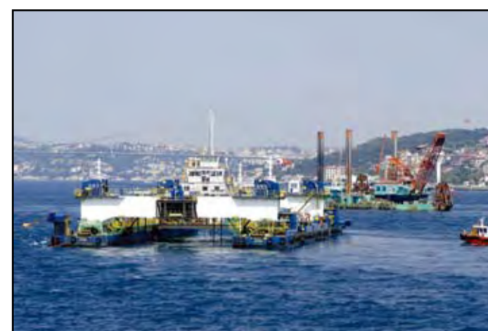
In what many hope to be a sign of increased bilateral cooperation, Japanese construction and engineering giant Taisei Corp. is taking part in the construction of a tunnel under the Bosphorus Strait, which will link the European and Asian sides of Turkey.
