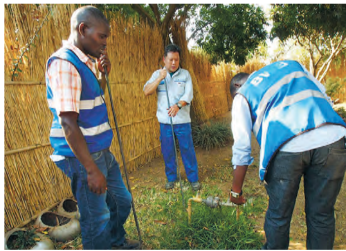
A Yokohama official and his African counterparts conduct a water leakage inspection in the Republic of Malawi. CITY OF YOKOHAMA
